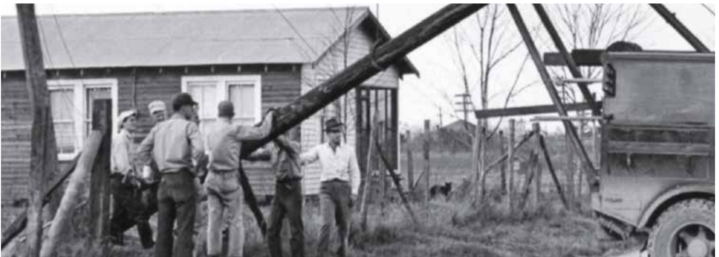
DEMCO began providing power in August of 1938, and now serves more than 119,120 meters in Ascension, East Baton Rouge, East Feliciana, Livingston, St. Helena, Tangipahoa and West Feliciana parishes.
