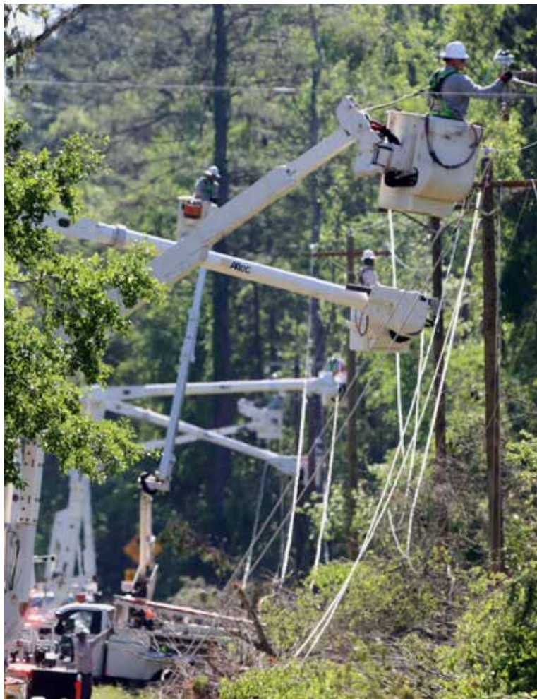
Demonstrating true cooperative spirit, DEMCO crews and mutual aid partners from fellow electric co-ops worked together to restore power after storm damage.
