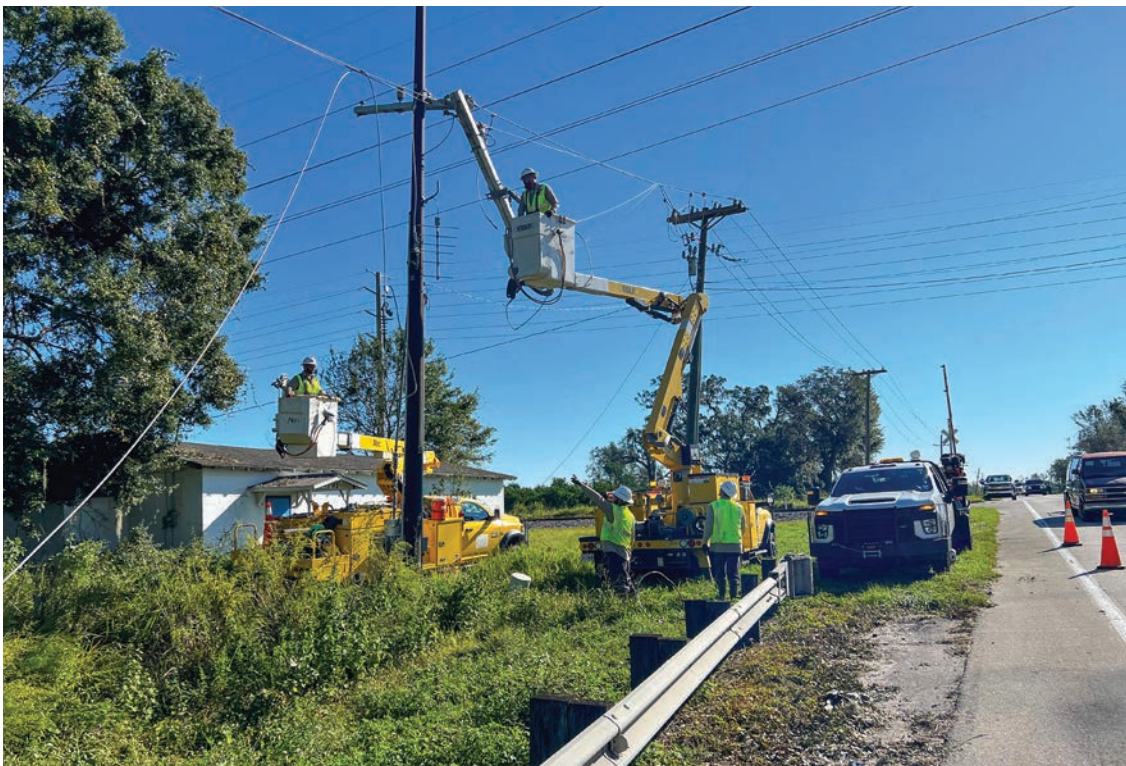
Claiborne Electric Cooperative crew members reattach lines on Peace River Electric Cooperative's power system in central Florida. From left are Andy Mills, Josh Dupree, Rocky Lachney and Ryan Beach.
