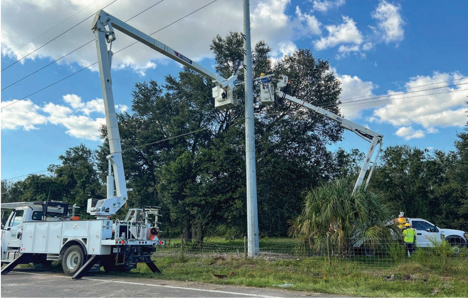
Lineworkers from Beauregard Electric Cooperative, left, and SLECA work together during power restoration following Hurricane Ian.
