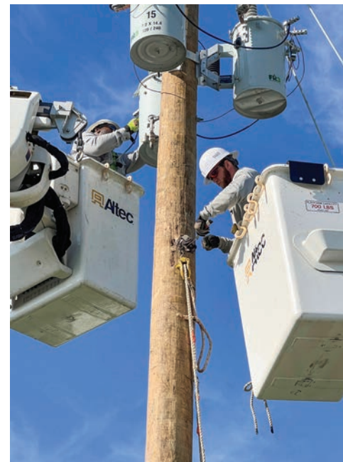
DEMCO's Orlando Hill, left, and Braden Owens rebuild a transformer bank serving a Florida dairy farmer.
