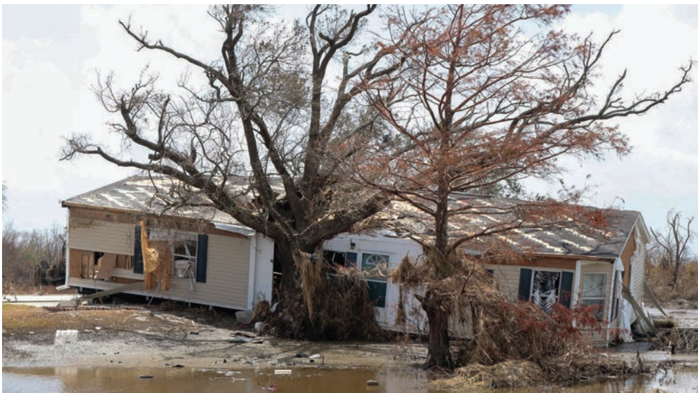
Winds of up to 150 mph flattened buildings and caused widespread destruction, including at this home in Cameron Parish. PHOTO COURTESY OF JEFF DAVIS ELECTRIC COOPERATIVE
