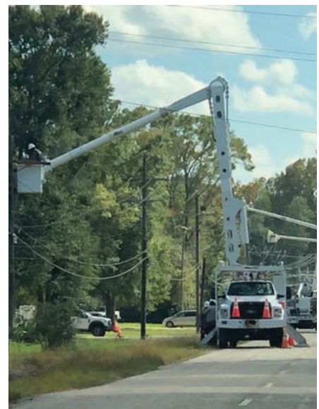
ABOVE: DEMCO crews and contractors work to restore power to consumer-members following Hurricane Delta.
