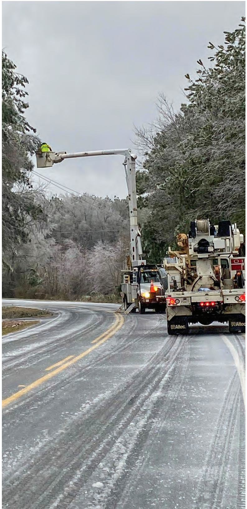
More than 100,000 power outages were reported throughout South Carolina on January 16 following Winter Storm Izzy. Cooperative crews descended on the region to help repair lines and restore electricity.
